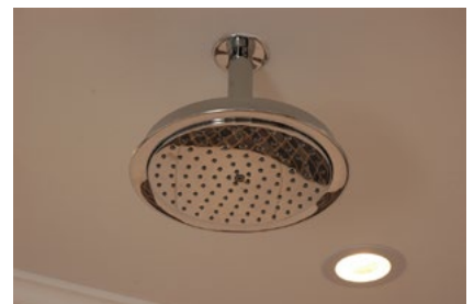
Ceiling mounted rainfall showerhead.
